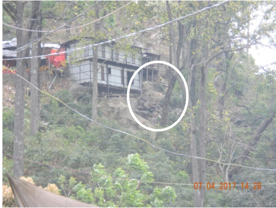
One more structure on the edge, the encircled portion shows stepping drain pipes emptying onto the slope
